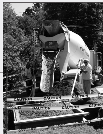
Concrete workers from S.D. Ireland prepare the base for the Old Soldier's move to the Museum grounds in August 2004.
